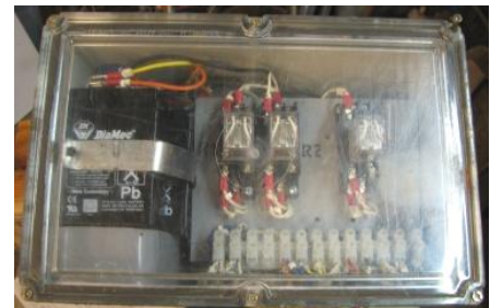
Electrical Control box – note all conductors are numbered
